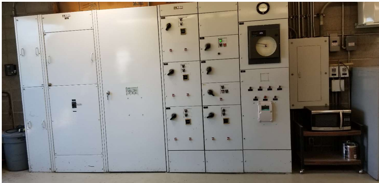
MCC LOCATED IN GARAGE AREA ABOVE DRY PIT
